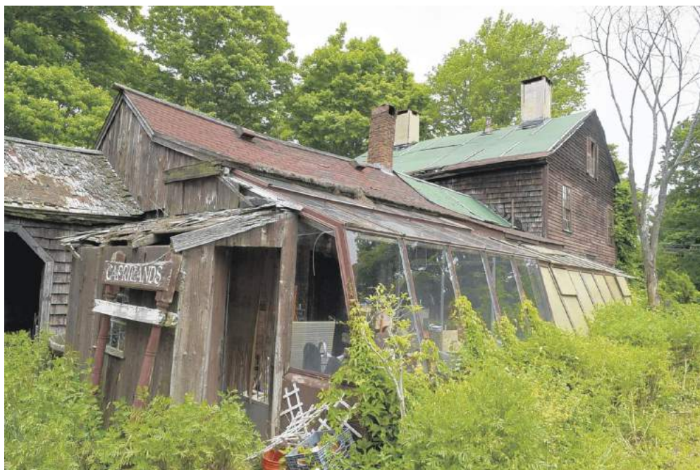
The 18th-century farmhouse at Caprilands Herb Farm has fallen into disrepair. (Jim Michaud / Journal Inquirer)
